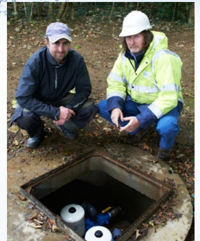
Rob Cook with WPT Technical Manager, Nigel Ponsford at the Papa Installation.
